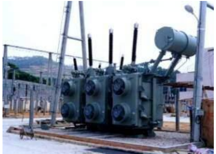
Power Transformer with 6 cooling fans Source: Siemens Transformers ETGZ
